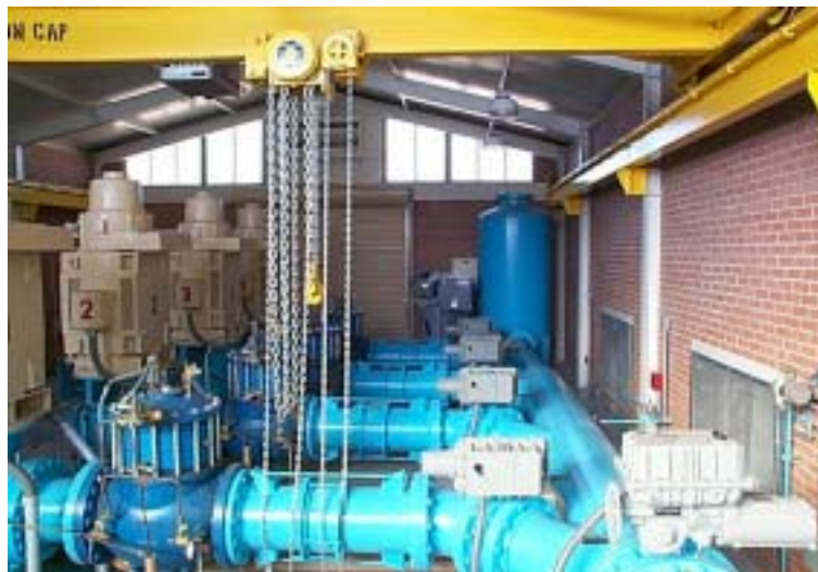
System pump station
