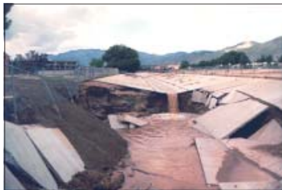
Drainage system failure
